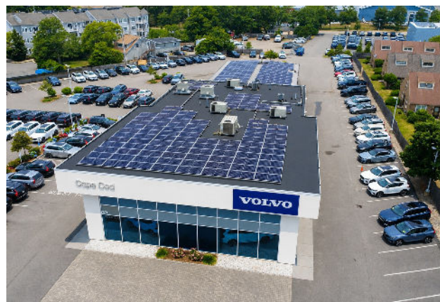
Volvo Cape rooftop solar
